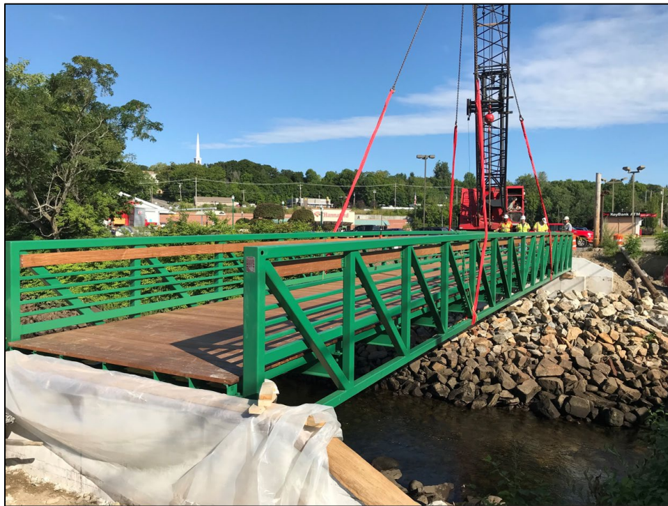
Figure 9. Installation of the Cobbossee Trail Multi-Use Bridge in downtown Gardiner using a single 110-ton crane for the 10-foot-wide, 76.5-foot span bridge.
